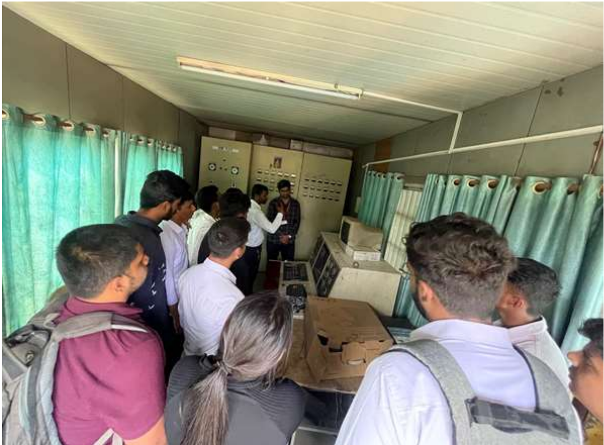
Control Unit of HOT Mix Plant
